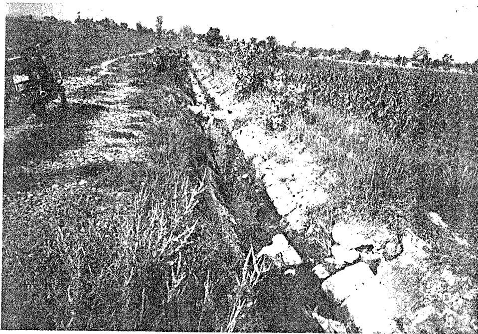
Photo – 5: Lined section damaged in branch - 1 Panchakanya Irrigation System
