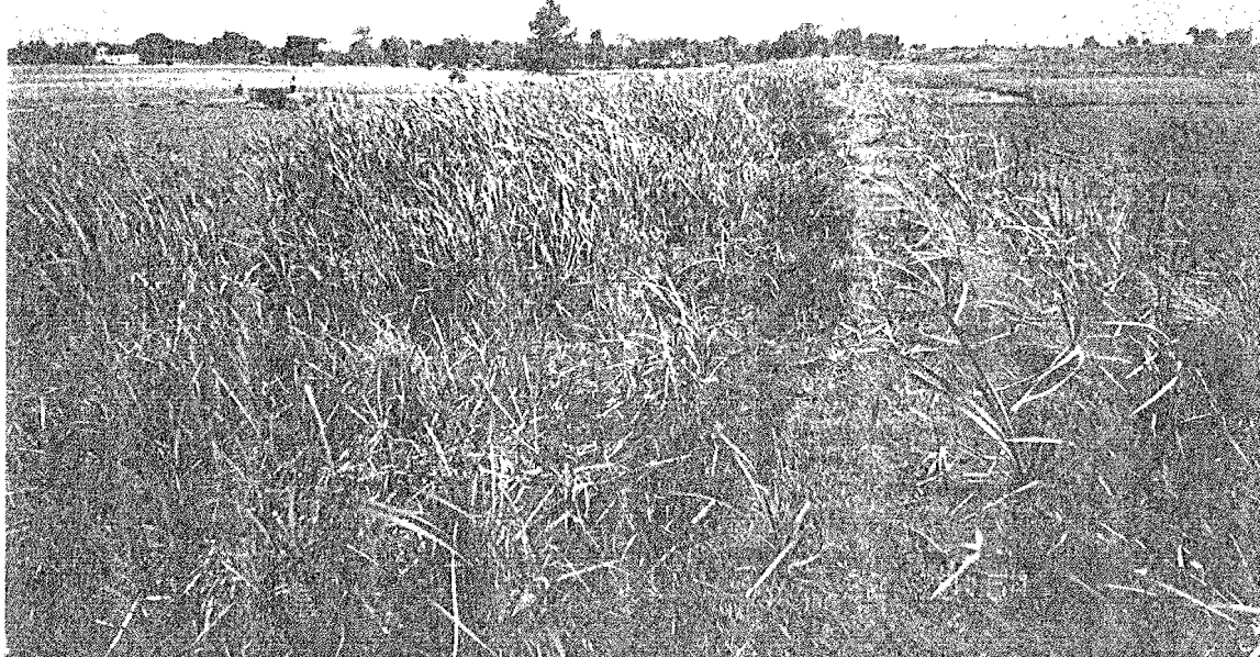
Photo - 30: Canal section covered by weed at tail end of Bishnuganj Nepal West Gandak Irrigation System
