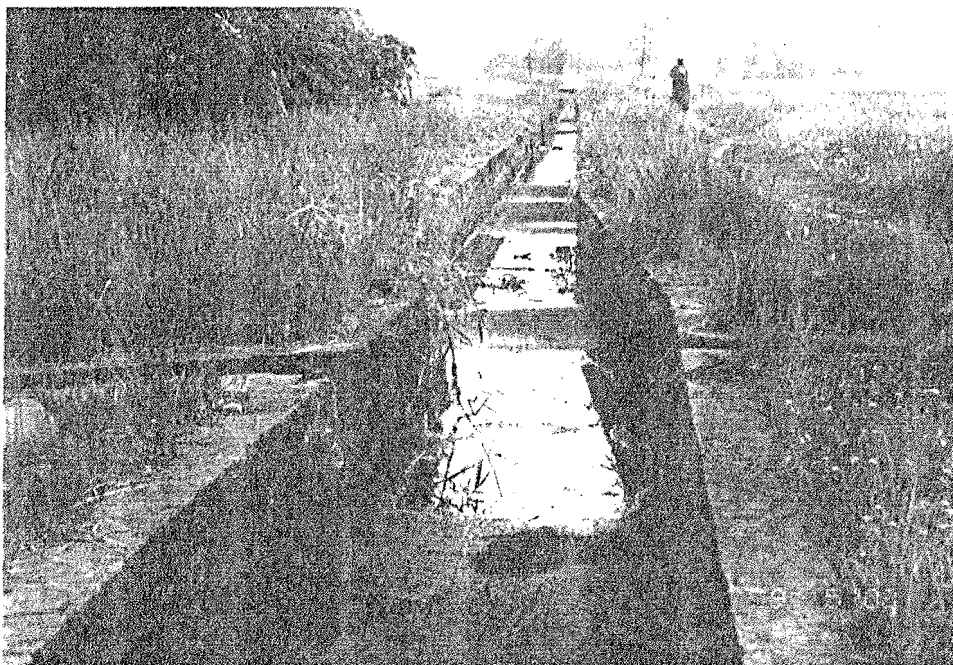
Photo – 15: Lined section with outlets (without control Structure) branch - 1 Khageri Irrigation System
