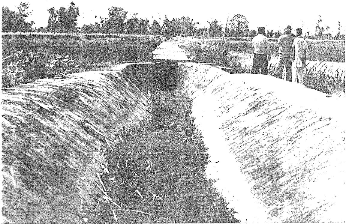
Photo – 28: IMTP's construction of aqueduct at Parsauni minor Nepal West Gandak Irrigation System
