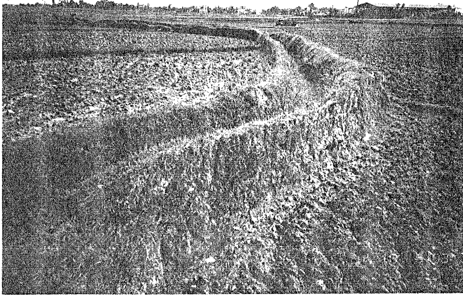
Photo - 9: Canal bank cut almost vertical at side (branch - 7) Panchakanya Irrigation System
