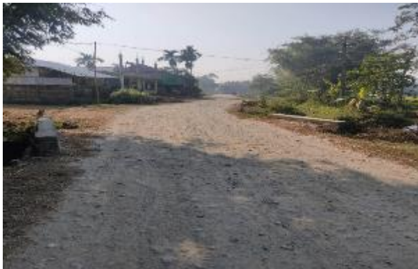
Road Condition Ch 2+080 to 2+290, Danalal Tole
